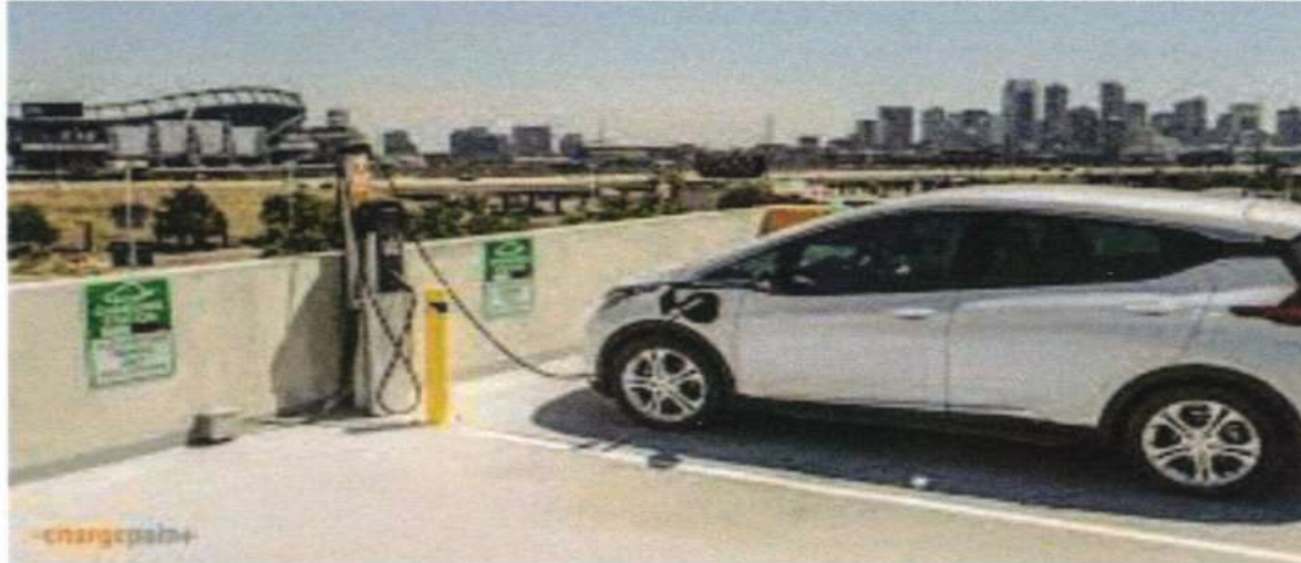
Electric vehicle charging
