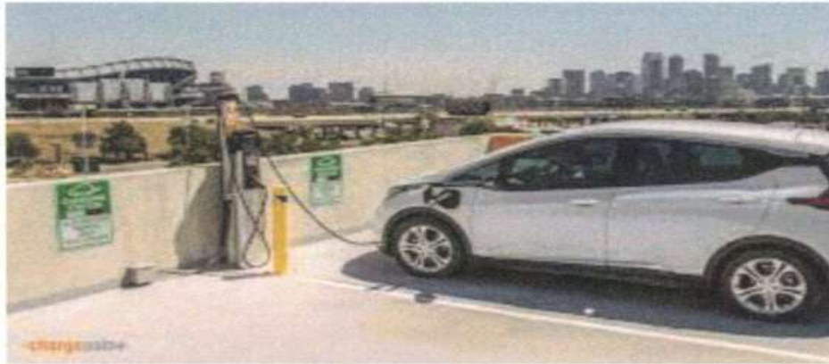
Electric vehicle charging
